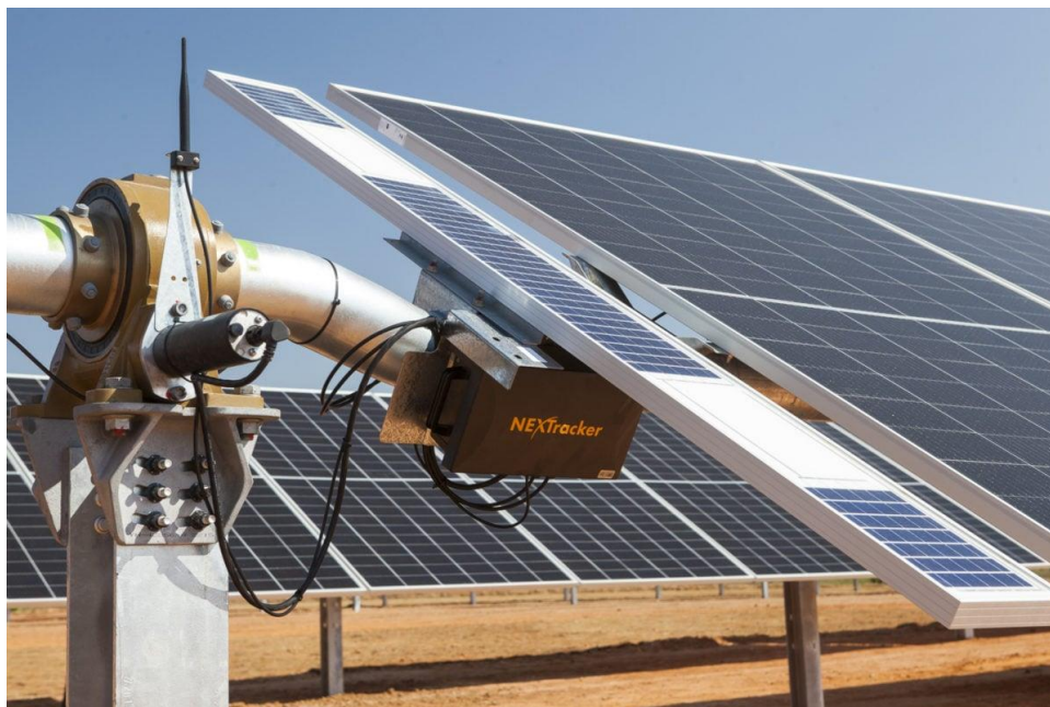
Note: NexTracker's software-enabled solar tracking solution
